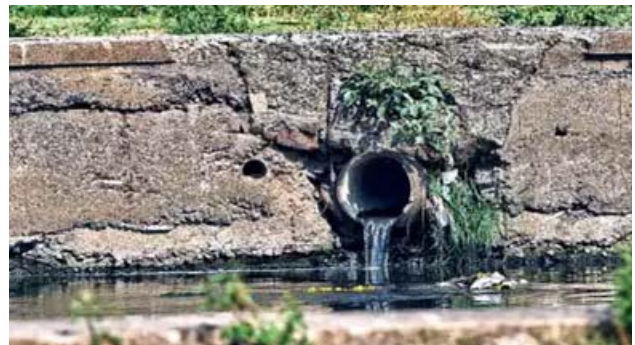
Untreated sewage being disposed in the River Channel
