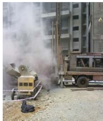
Dry borewell with no connectivity with the aquifer hence not the right place for attempting to recharge the groundwater
