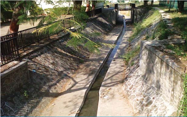
Photo of Modified stream channel, where the flow alignment is through paved concrete channel
