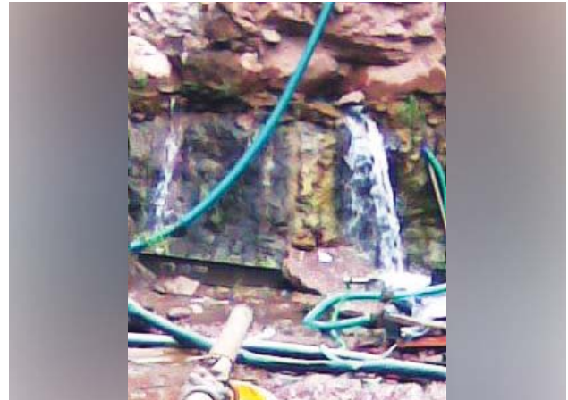
Groundwater flow encountered in excavation of basement which needs to be pumped out during and after the construction is over
