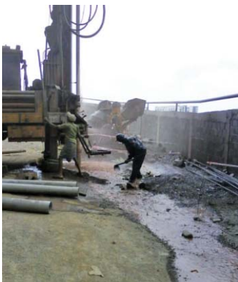
Photo of a borewell drilled with a good connectivity to the aquifer and hence good place for attempting to recharge the groundwater
