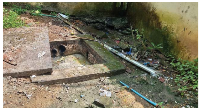
Fig 3: A badly managed grease interceptor
